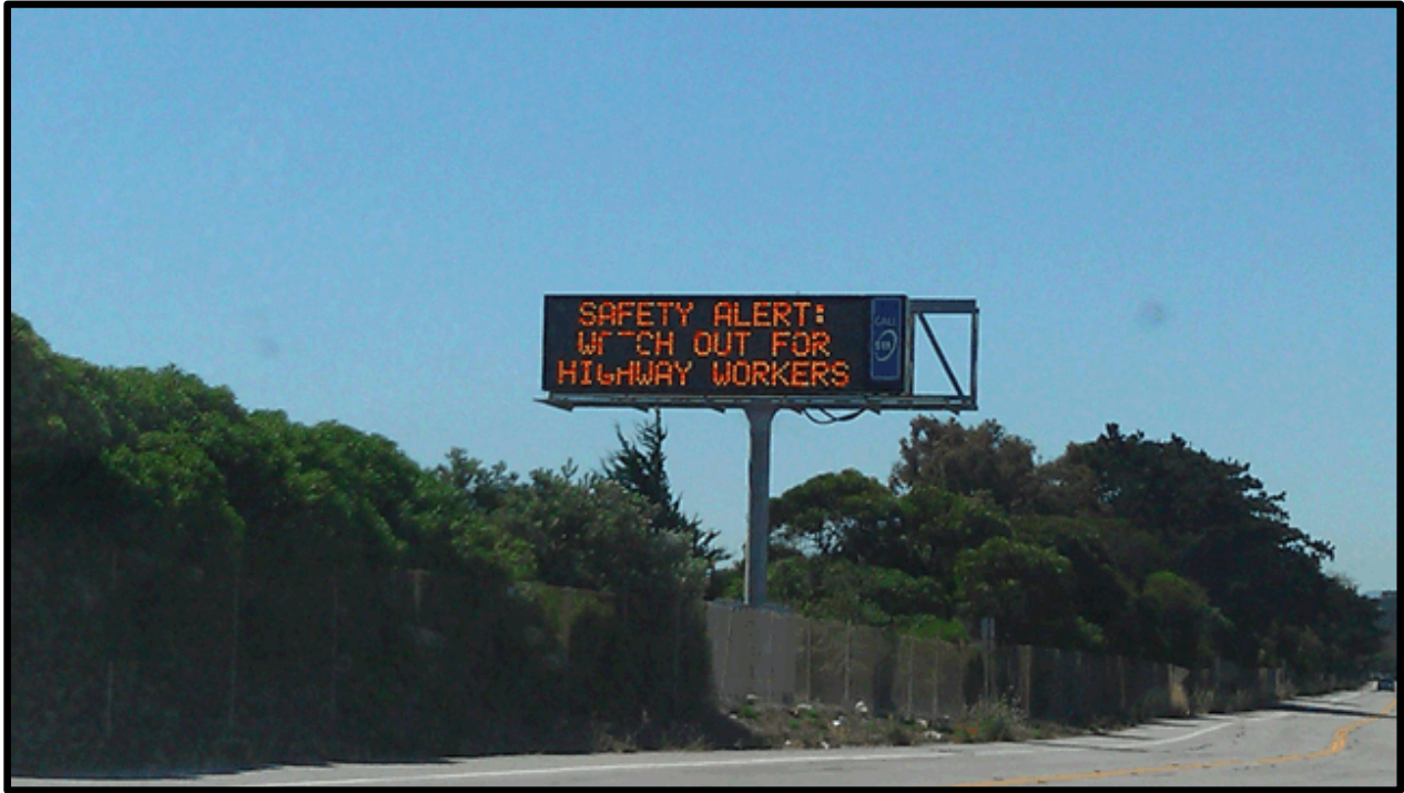
Photo 6: Example of a malfunctioning CMS
