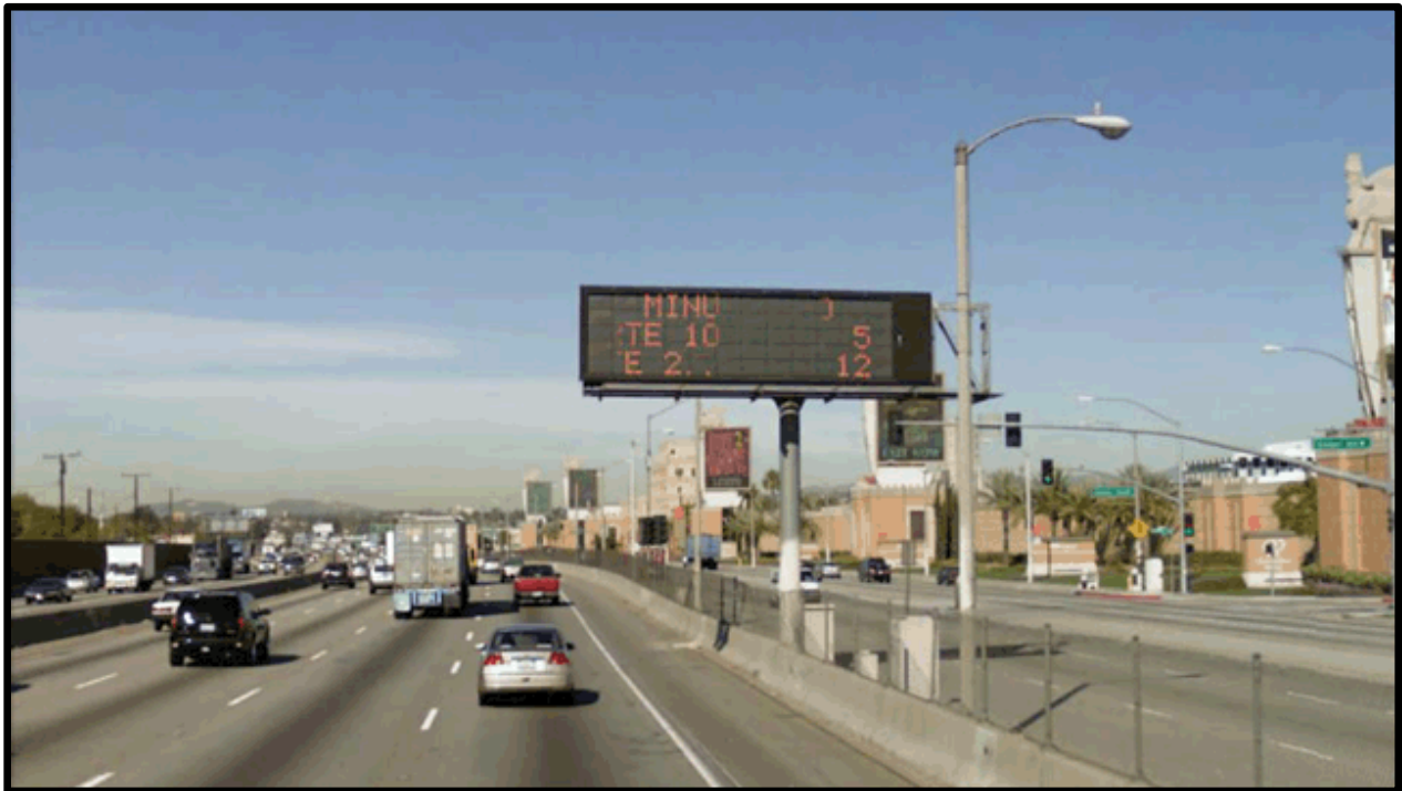
Photo 5: Example of a malfunctioning CMS
