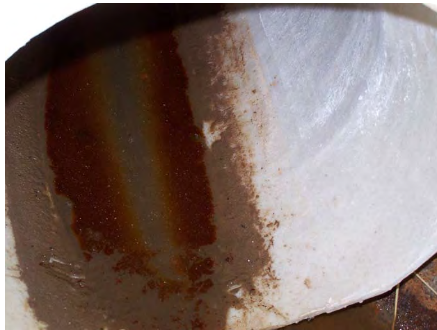
Figure 2. Residue on water surface in pipe at Site 2 between stormwater events, 24 days after installation.
