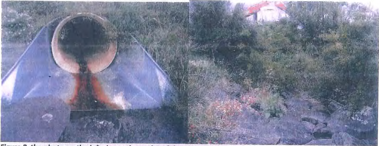
Figure 2 the photo on the left shows the outlet of the pipe that was replaced in the summer of 2008 using the CIPP technique. This is the location where sample A-1 was taken. The trickle of water that left the culvert under the eastbound lanes of I-88 traveled along the rocky ditch shown in the photo on the right. The location of the inlet to culvert A is marked by the orange scaffolding and the white trucks.
