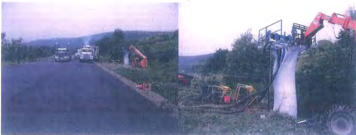
Figure 1 The photo on the left shows the scaffold holding the liner in the inlet to culvert A. The diesel powered furnaces to heat the curing water are on the trucks. The photo on the right shows the hoses that re-circulate the water.
