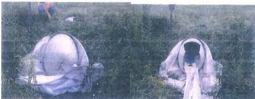
Figure 11 Photo on the left shows the lining in culvert D before it has been cut. Photo on the right shows the cut lining. The blue plastic tubing used to convey the heated water to the end of the lining in situ can be seen in this photo.
