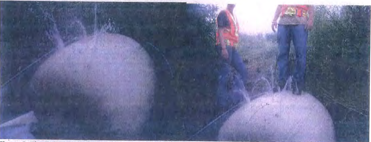
Figure 3 The lining in the outlet from culvert A after curing complete and holes were made in the bag to collect water (A-4). The photo on right shows water leaking from the holes before the end was cut.
