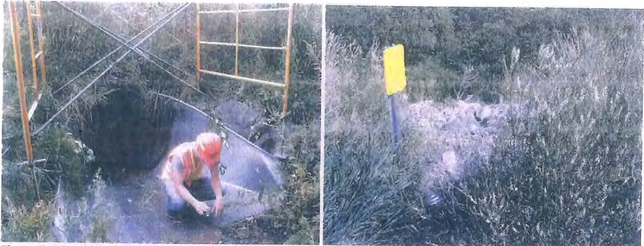
Figure 5 TCI taking water sample from upstream of culvert B. Scaffolding is already in place. Photo on the right show the outlet from culvert B.
