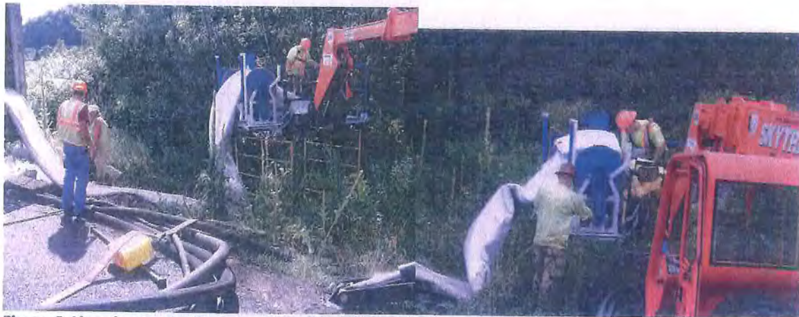
Figure 6 Liner is unrolled from truck and fed through the specialized equipment on top of the platform.
