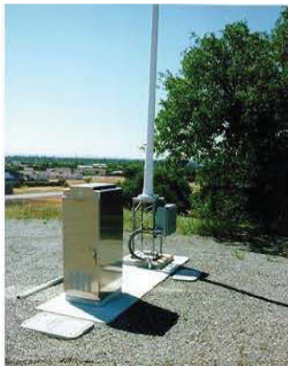
Extended Coverage HAR Installation - Redding
