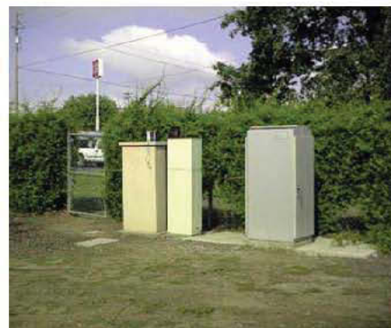
Site Cabinets (HAR Far right) – Red Bluff
