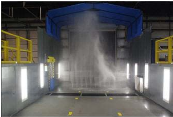
Undercarriage/ Wheel Wash Spray Bars
