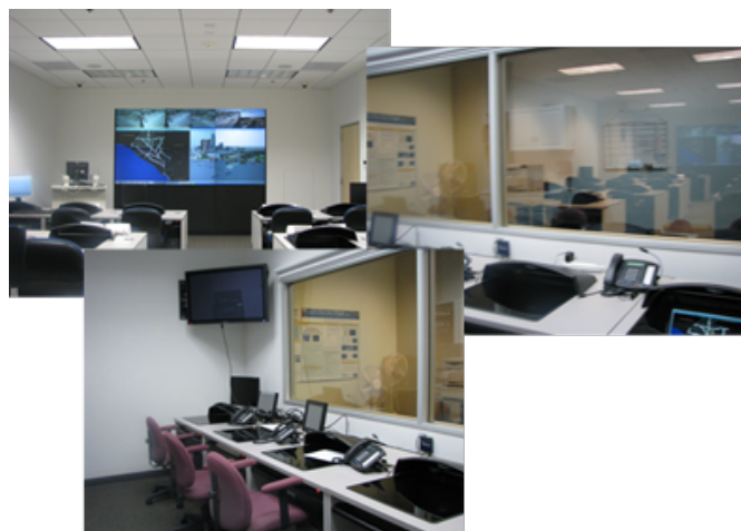
Image 1: Traffic Management Center (TMC) Training Simulator facility as installed at University of California Irvine (UCI).
