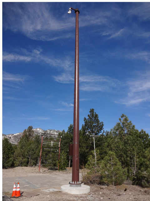
Picture 2: Internal-Type CLD System, US-50 at Meyers
