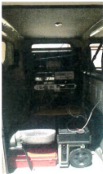
Image 2: Photos of the server racks holding the equipment
